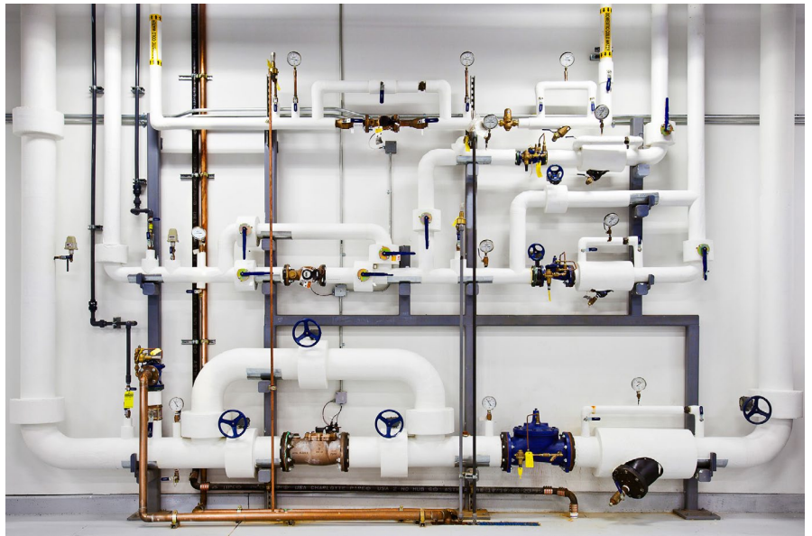
We keep pipes like these at our Douglas County, Georgia, data center ready with highly pressurized water in case of a fire.
